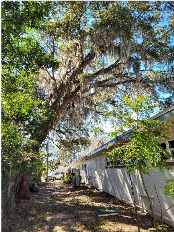
Leaning Over Building
