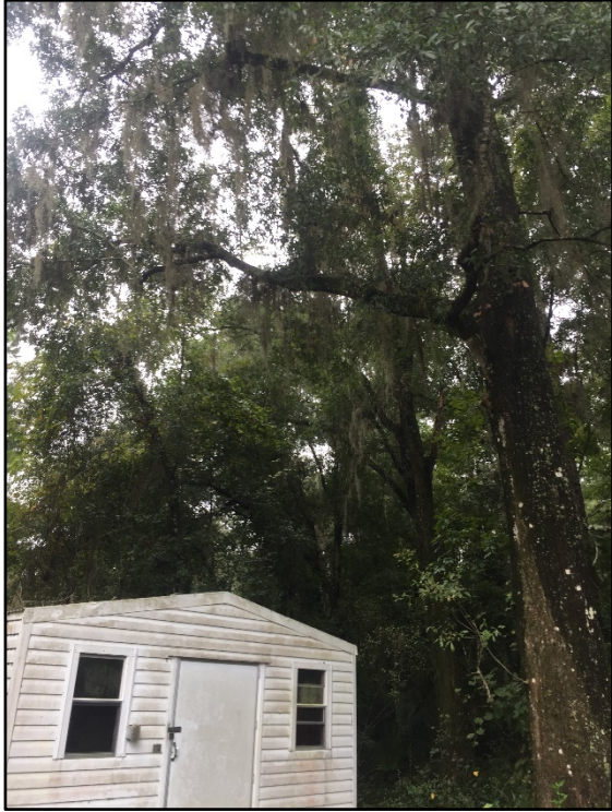
Image One: Tree one, notice dead branches on top the roof.
